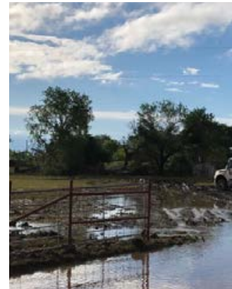
REPAIRS IN MEDINA COUNTY FOLLOWING THE APRIL 28 TORNADO AND RECORD-SETTING HAIL EVENT.
